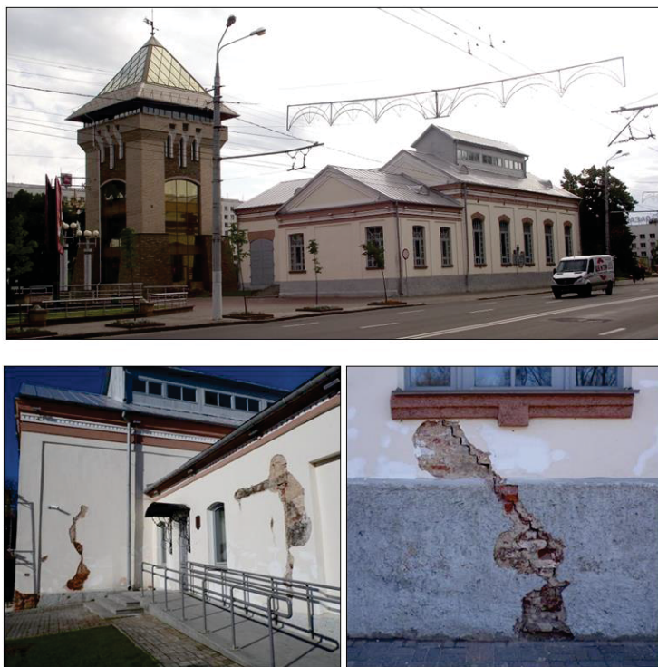
Fig. 7. Building of the first power station in Vitebsk (1897–1898) along Frunze Avenue in the historic part of the city and cracks in wall structures resulting from vibrations during the movement of urban transport (2016) [25]
