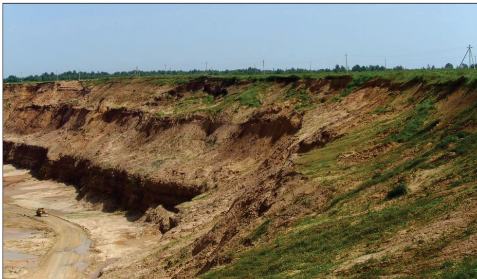
Fig. 3. Southern wall of the Galevo open pit for dolomite mining with numerous rockfall-landslide areas (May 2010). Photo by A.N. Galkin
