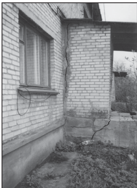
Fig. 9. Cracking in a residential building on the Lenin street, 101 in Liozno (Vitebsk region) as a result of heaving of moraine soils (2005) [10]
